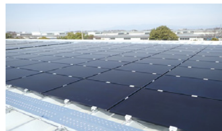
Solar panels installed at the Nitta Plant around 160 kW
