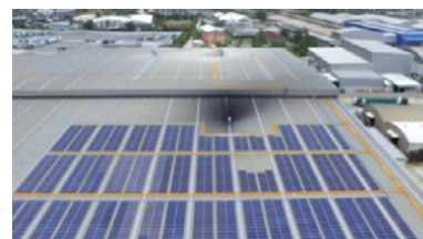
Solar power generation panels installed on the plant roof
