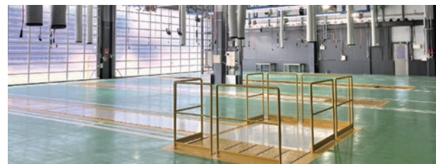
Floor lifts equipped with fall-prevention mechanisms
