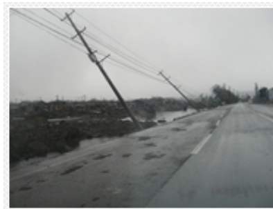
A view of the extent of the damage
