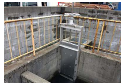
Blockade dam for preventing abnormal drainage
